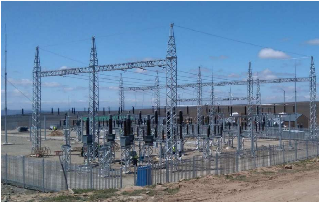
Figure 12: Example of High Voltage Substation
