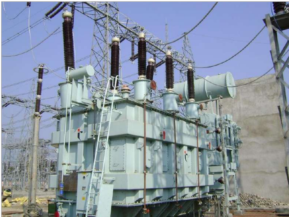
Figure 11: Example of Medium Voltage Transformer (Source: https://www.ulaginoli.com/ )
