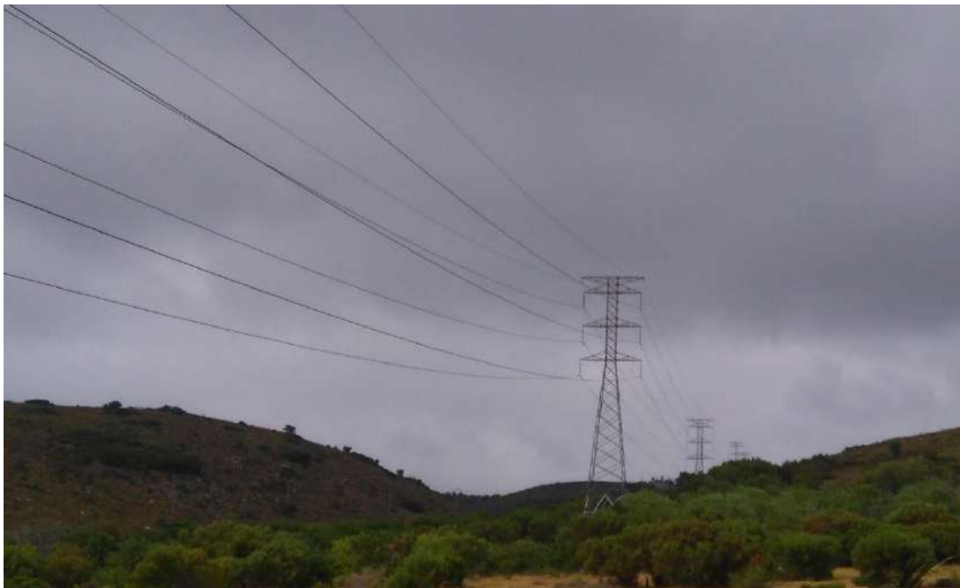
Figure 16: Example of a 132kV transmission line
