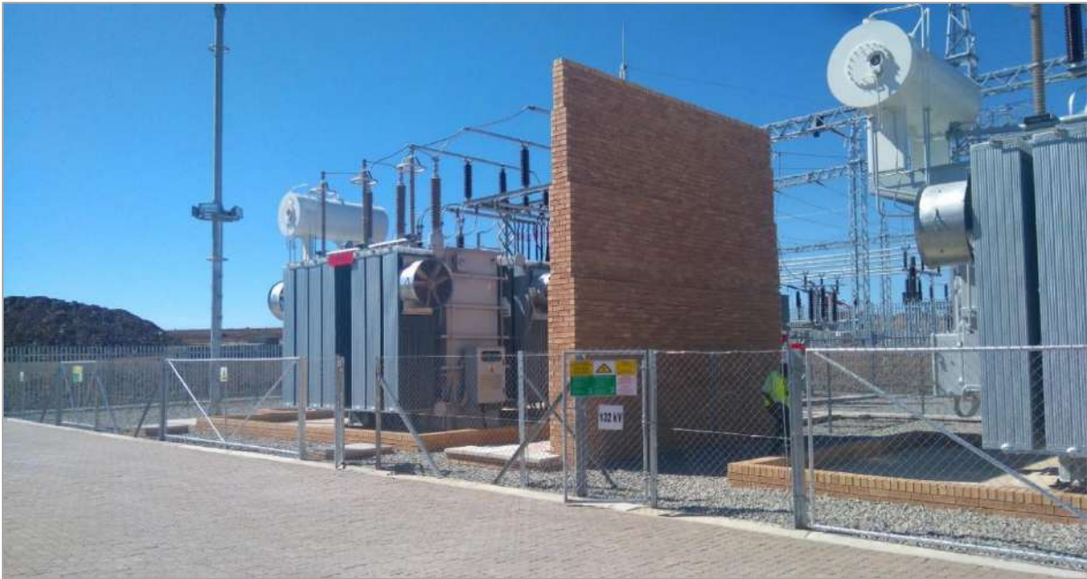
Figure 13: Example of High Voltage Transformers
